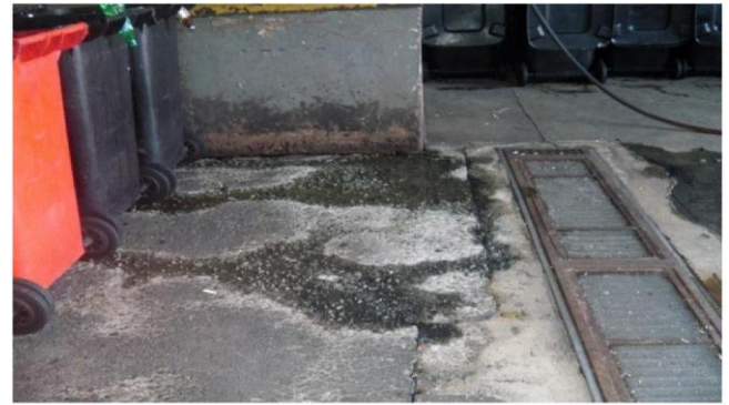
Plate 4.5: Damaged concrete flooring
