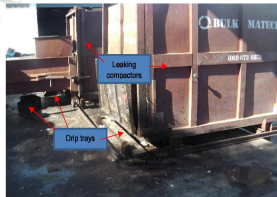
Figure 4.13: Leaking compactor and overflowing drip tray
