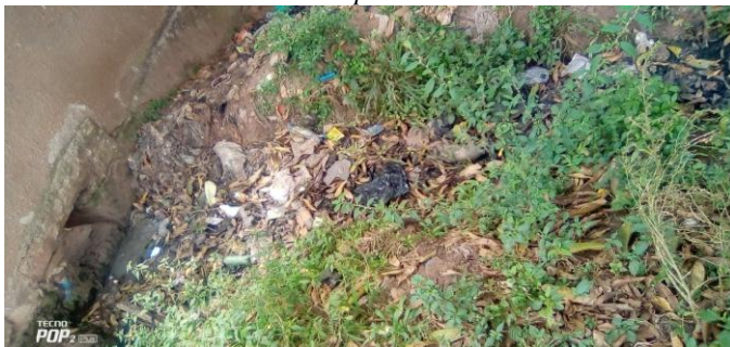
Plate 4.4: Drainage channels clogged by waste around Thorban area (Source: Field photo)
