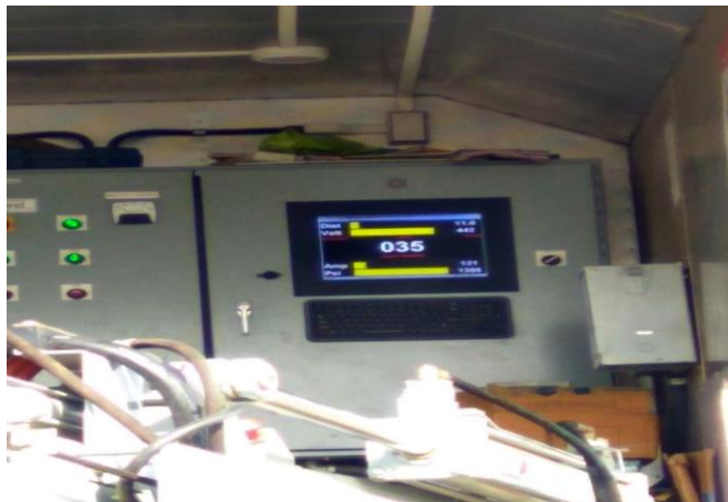
Weld management system
